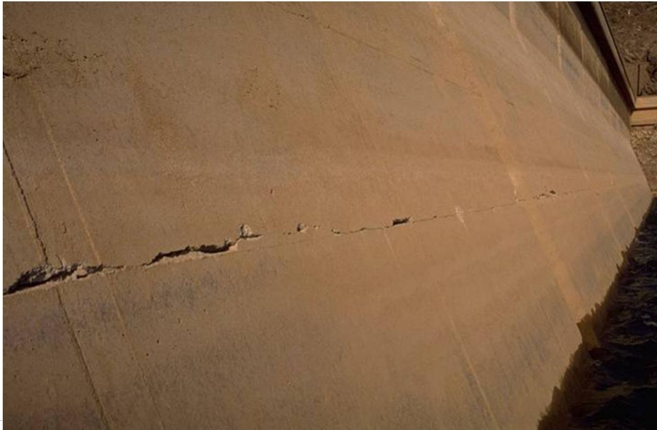
Crack at upstream face of Sefid Rud buttress dam
