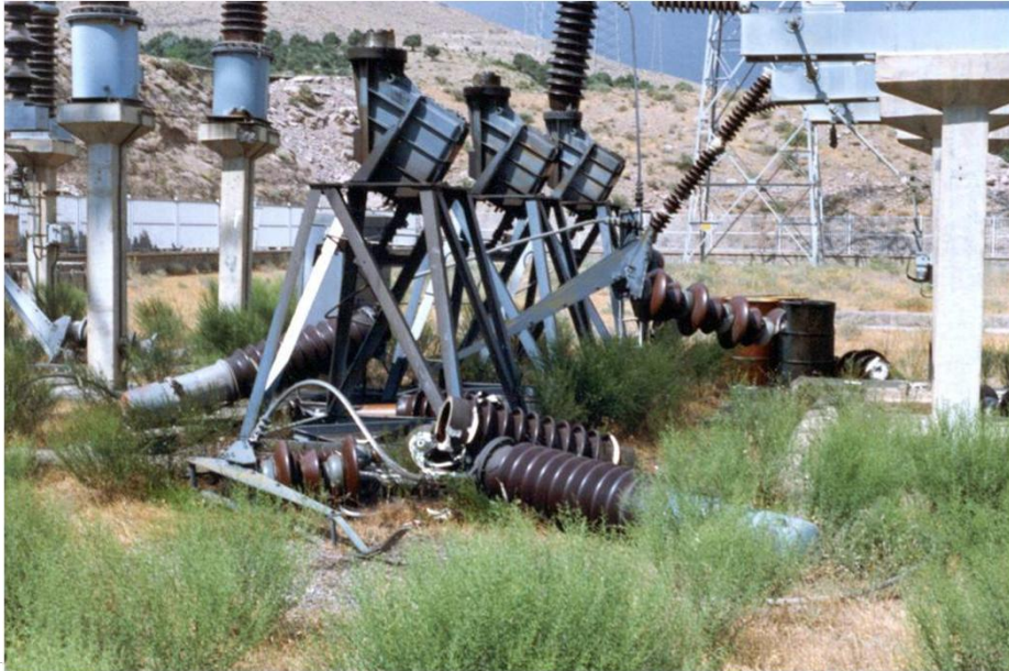
Damaged switchyard on fill, Sefid Rud dam
