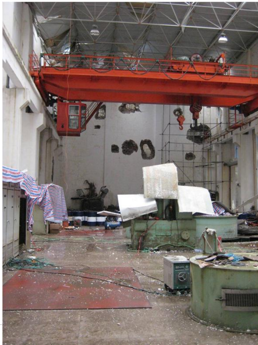
Rockfall damage of surface powerhouse and equipment, Wenchuan earthquake, 2008 (China)
