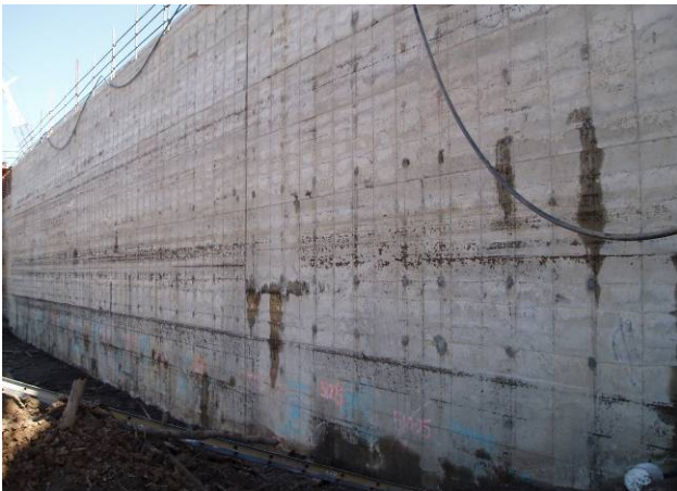
Figure 23. View from the upstream face of the Eidsvold Weir prior to commencement of the waterproofing activities.
