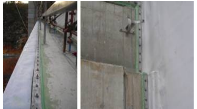
Figure 21. The seal over the primary spillway, along the upstream plinth, and at the outlet tower is watertight against the water pressure, and was tested at 240 m head.
