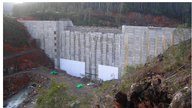
Figure 16. Installation of the anti-puncture geotextile on the lower part of the panels.
