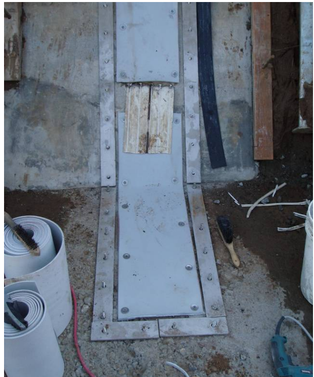
Figure 26. View of the support layer at the foot of the vertical joint. The waterstop can be seen emerging from the RCC body.
