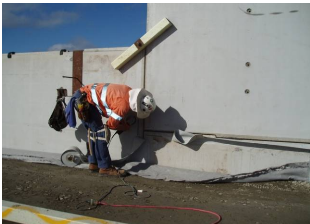
Figure 5. View on the inside face of the panels, showing the PVC geomembrane embedded in the grout cap.
