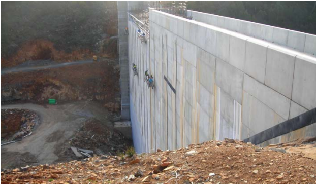
Figure 17. The black band of geonet along the plinth at the right abutment collects and conveys drained water to the discharge points.
