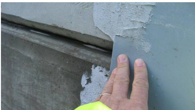
Figure 15. Additional sacrificial layer of geomembrane spanning across a joint providing support to the main geocomposite.
